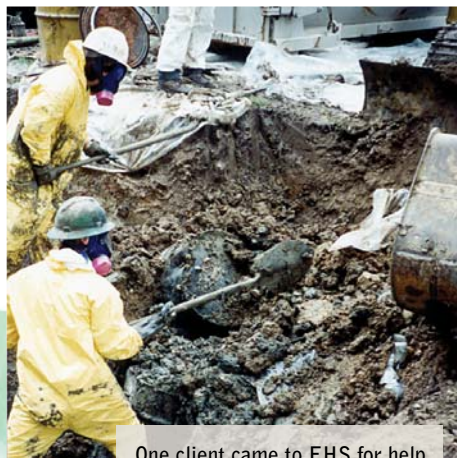
One client came to EHS for help after finding that a previous owner had buried 200 drums of toxic waste on their property.
