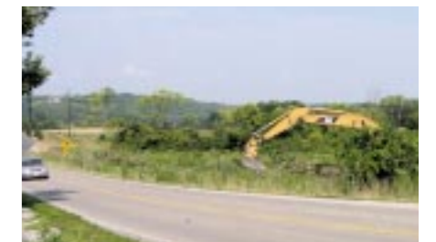
Preparations are being made to complete roadway improvements around the Mound site's perimeter.
